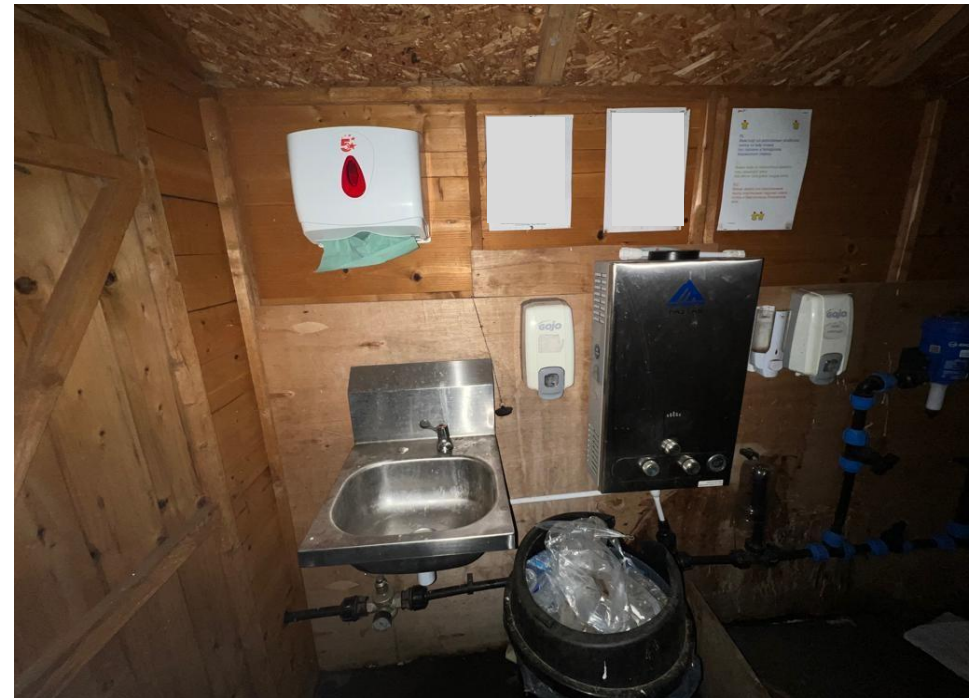
Provision of hand washing facilities and hand sanitiser.
