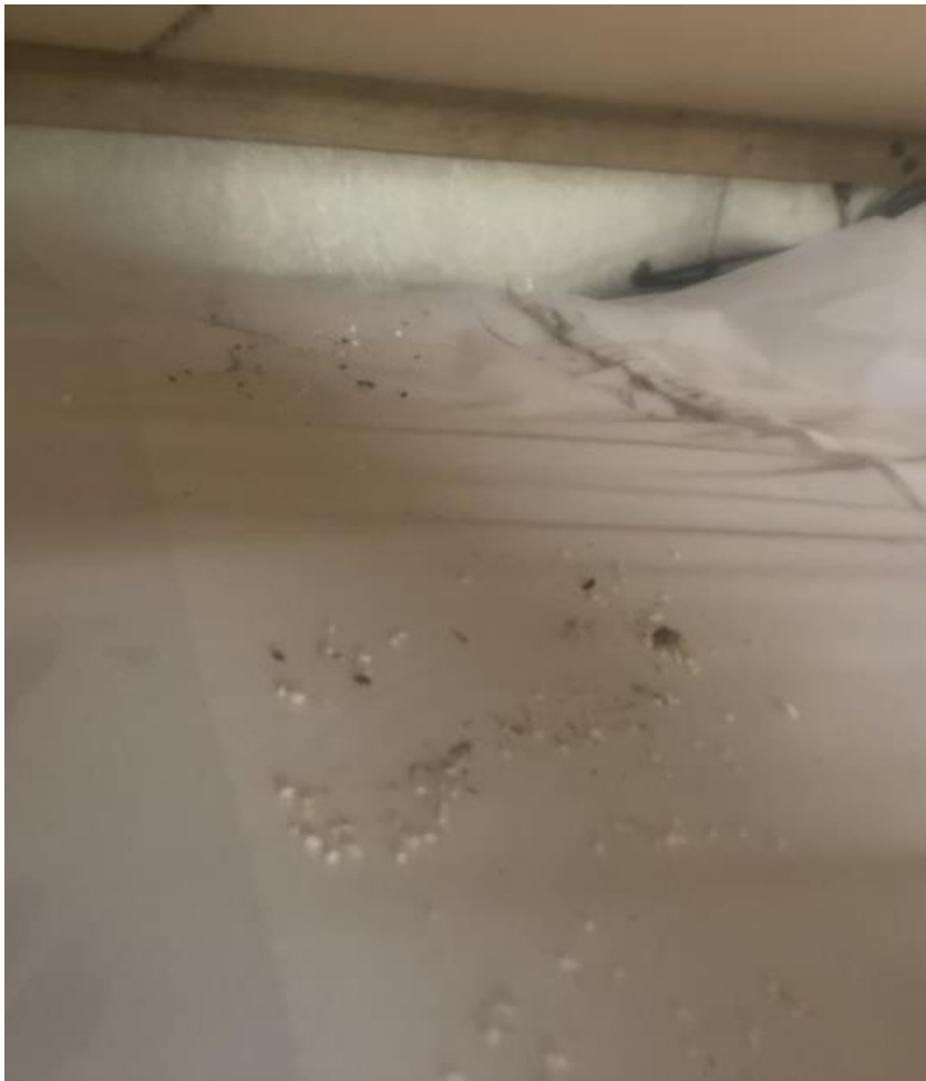
Mouse droppings in roof space
